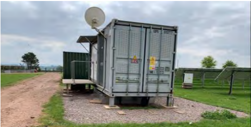
Photo 21 and Insert 7: Typical Tracks and Inverters
