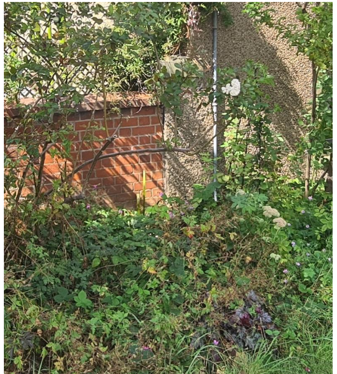
Figure 27 – The gate pier has been rendered here, but its form and the cap are still evident.
