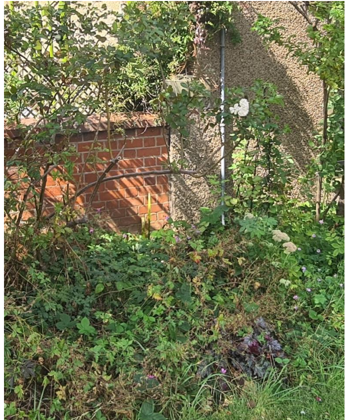
Figure 27 – The gate pier has been rendered here, but its form and the cap are still evident.
