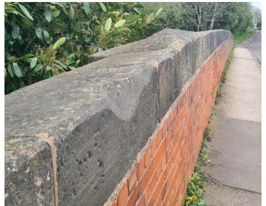
Figure 32 – Worn coping stone (Zone 1)
