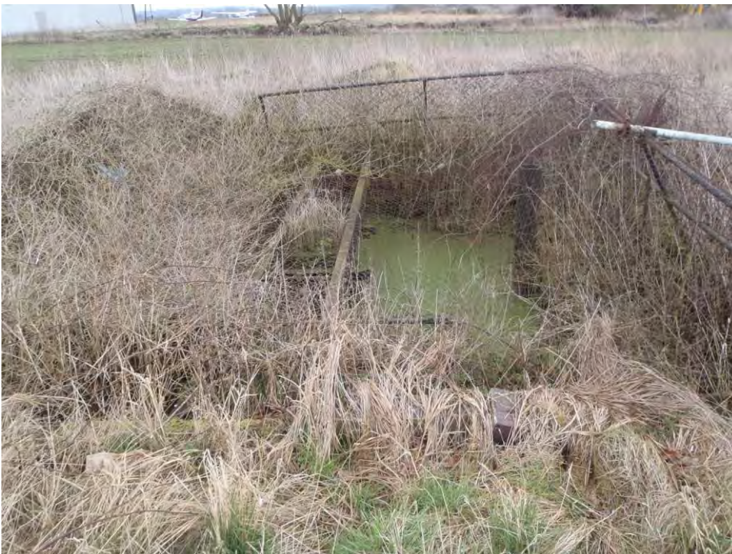
Photo 6 — Abandoned structure associated with sewage works. Algae present on surface water.
