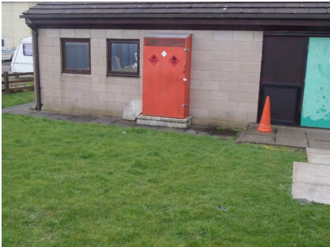
Photo 12— Flammable liquid and gas storage on business park.
