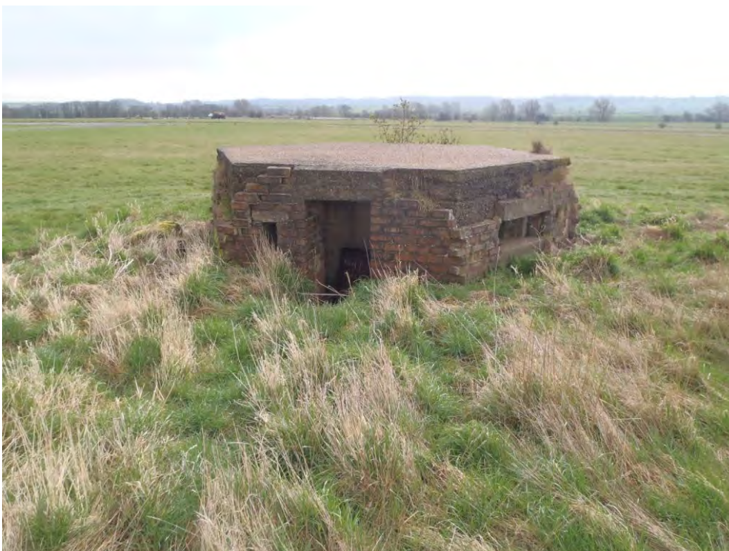
Photo 2— Grade II listed pill boxes found across Airport site in various states of disrepair
