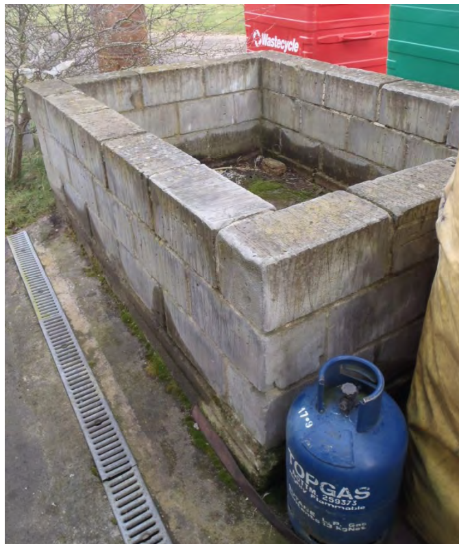
Photo 4 — Historic tank bund with waste Propane gas canister.
