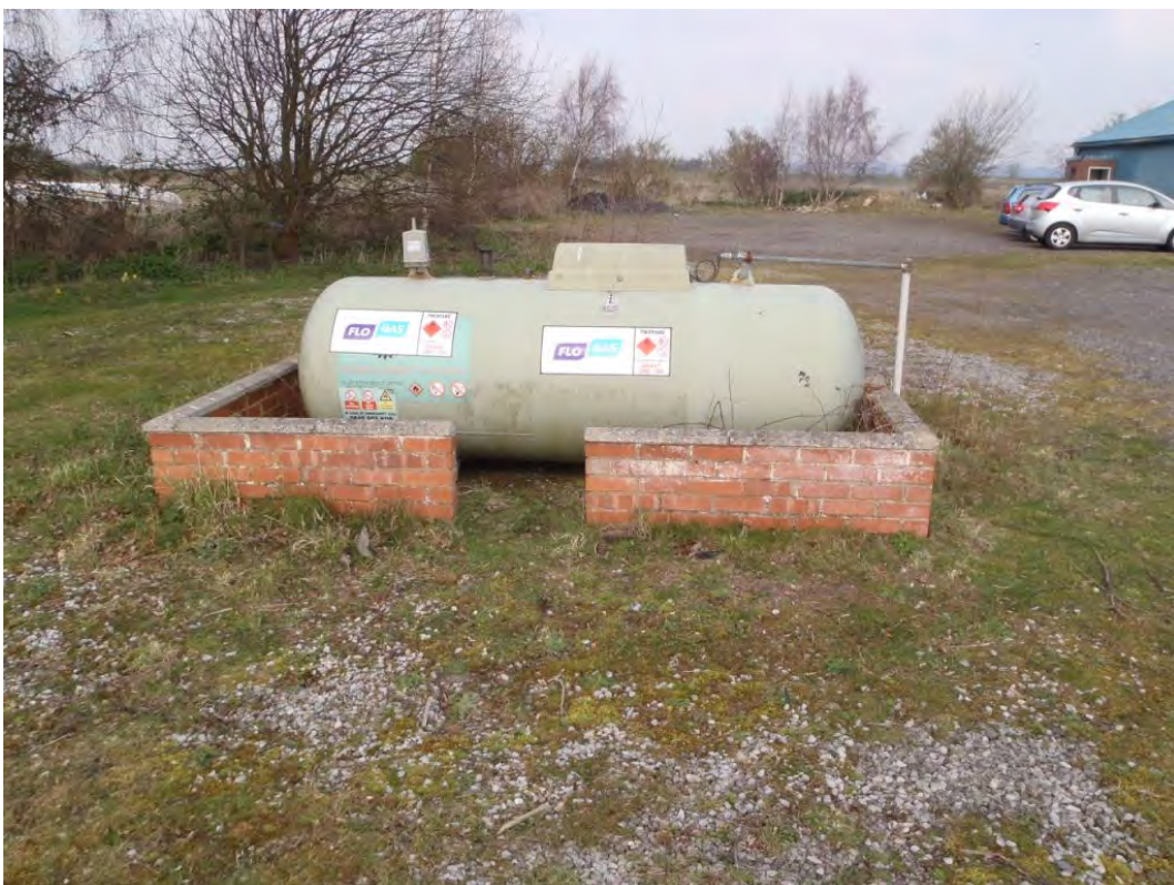
Photo 16— Propane gas tank in restaurant car park.
