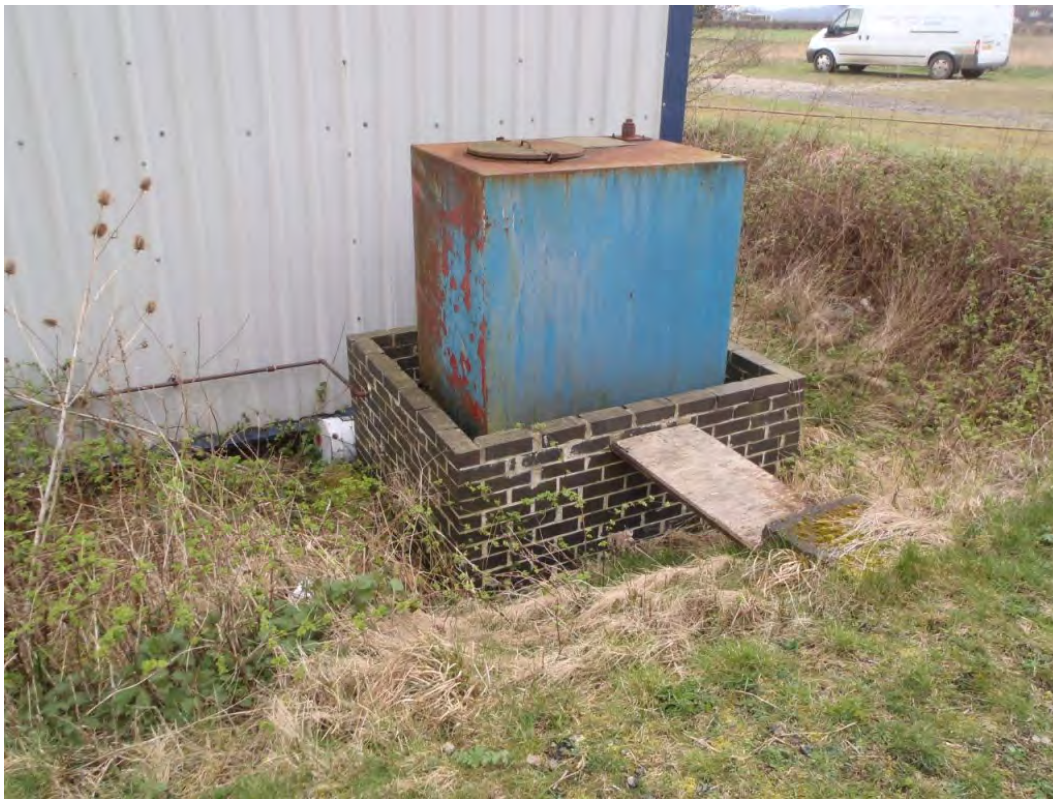
Photo 1— Historic bunded AST of unlabelled use located outside the aircraft hanger.
