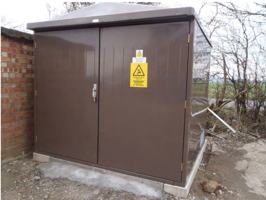
Photo 14— Electricity substation on Tollerton Business Park
