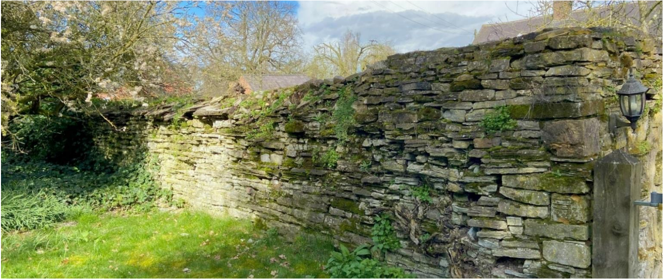
Figure 17 – Walls using what is thought to be medieval stone (Palace Curtilage Walls)
