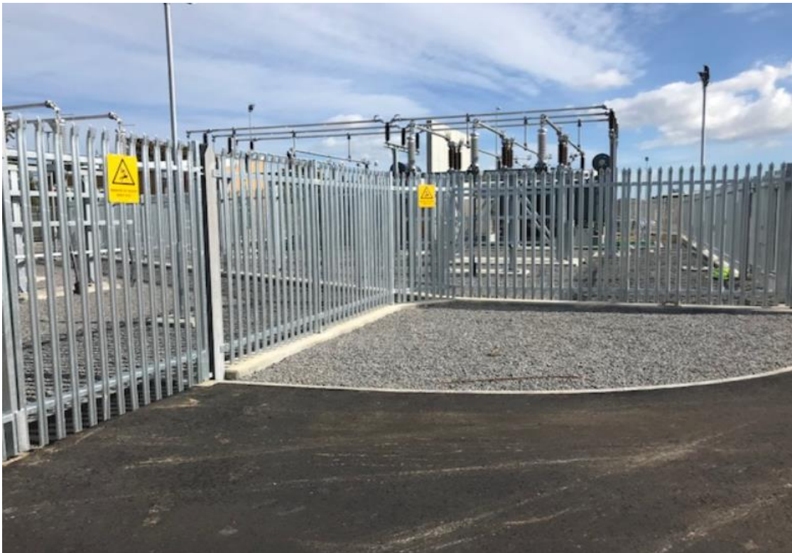
Typical DNO substation complex fencing
