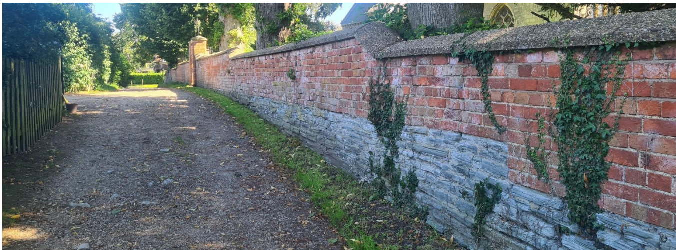
Figure 14 - Pathway and Wall Adjacent to St John of Beverley Church, Church Walk, (Zone 1)
