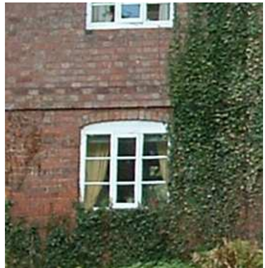
Tripartite timber casement window with segmental header and arched brick lintel (Garden House).
