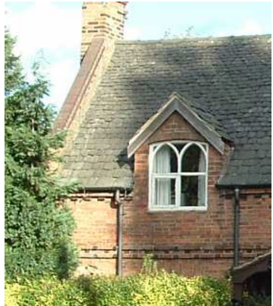
Side hung timber casement window with tracery style glazing bars; parapet gable, corbelled eaves and decorative string course (Foxglove Cottage).
