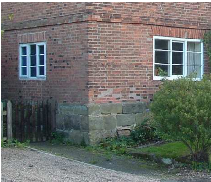
Stone plinth, Flemish bond brickwork and tripartite Yorkshire sash windows (The Cottage)
